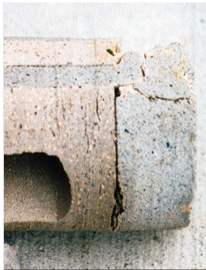
Photo 1. When a collar joint is filled with mortar, voids and cracks are the inevitable result.
