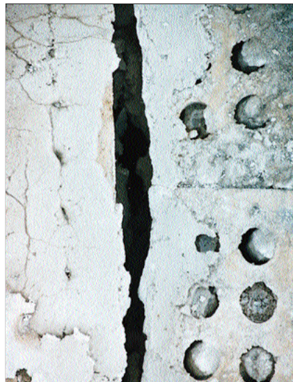
Photo 2. When a wall is designed with a collar joint that was not specified to be filled solid, what results is a space filled with mortar extrusions.
